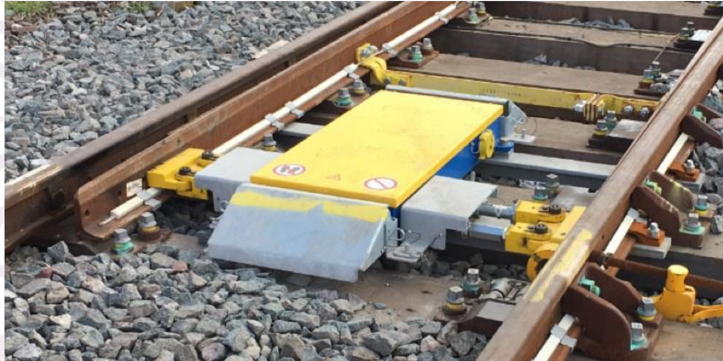
Figure 8 - Point machine installation
